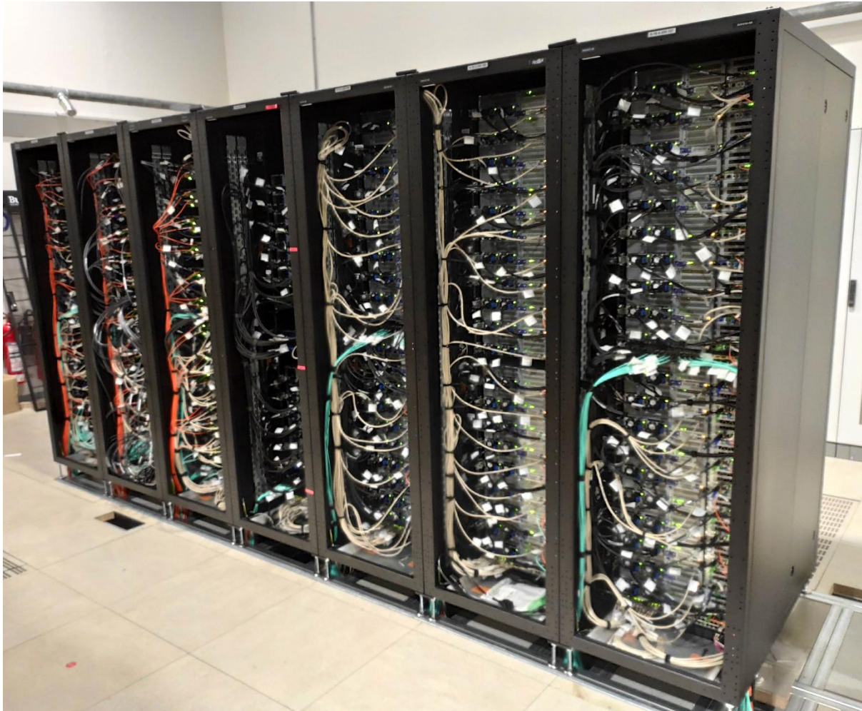
Figure 2: Photo of the JUSUF installation in the data centre. Please note that the rear-door heat exchangers have not yet been installed at the time the picture was taken.
